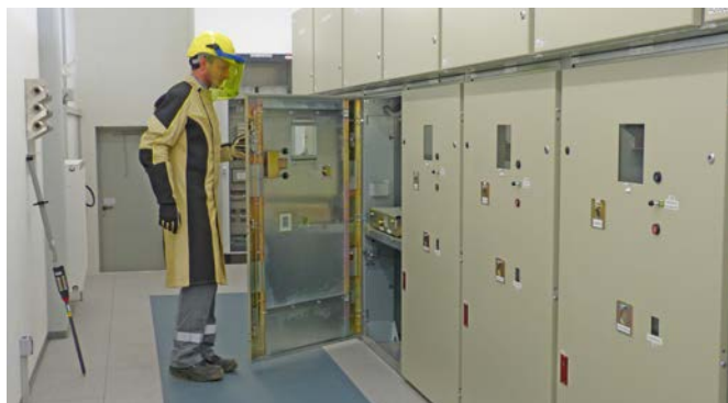
Switch room with insulating mat fitted.
