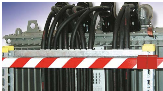
Barrier in a transformer station.
