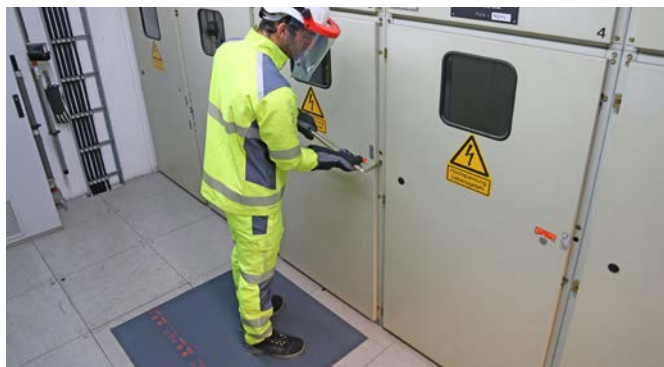
Switch room with insulating mat fitted.
