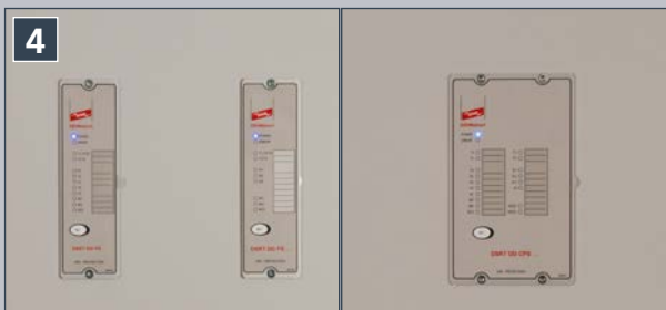
Detection devices are installed at the front of the switchgear assembly and LEDs indicate the current status of the system.
