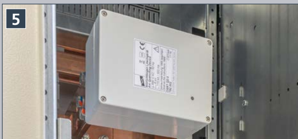
Quenching devices are preferably positioned in the vicinity of the supply switch.
