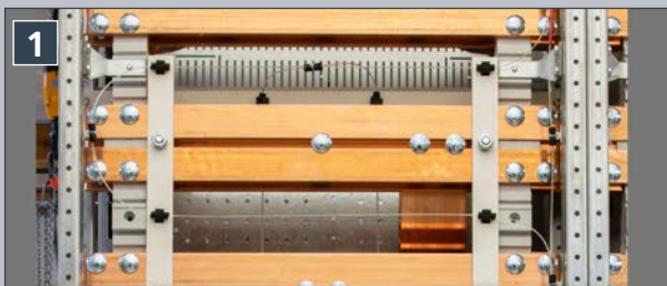
Fibre optic sensors are installed to detect the arc fault along all live parts of a switchgear assembly where ignition of an arc fault is to be expected.
