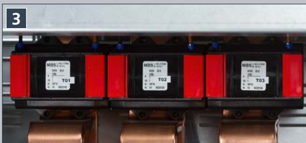
Current transformers detect the overcurrent resulting from an arc fault. They are positioned upstream of the incoming circuit breaker.
