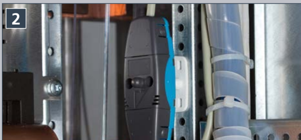
Optoelectronic sensors monitor a large area and, like the fibre optic sensors, detect arc faults in the vicinity of the active parts.
